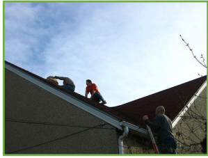
Top1: Three men are working on a roof . Top2: Two men sitting on the roof of a house while another one stands on a ladder .
