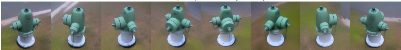
a green fire hydrant with a tag on it
