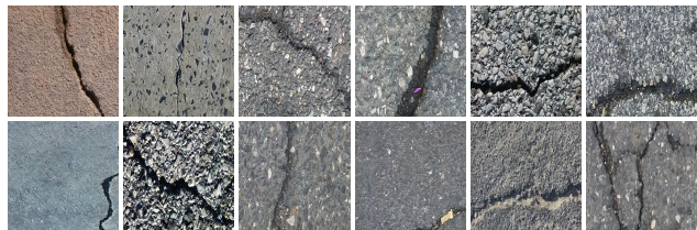
Figure 5. Representative crack images from the Crack500 dataset.
