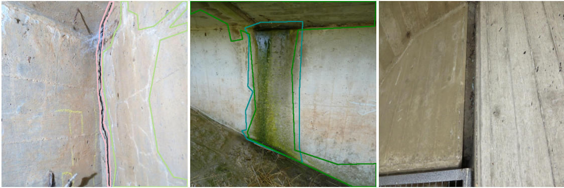
(b) Crack vs. Alligator Crack , Weathering vs. Wetspot , Restformwork covered with concrete slurry (no ground-truth annotation for better visibility).
