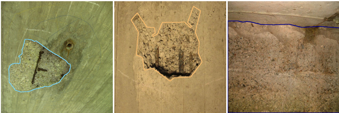
(c) Spalling , Rockpocket , Washouts/Concrete corrosion .
