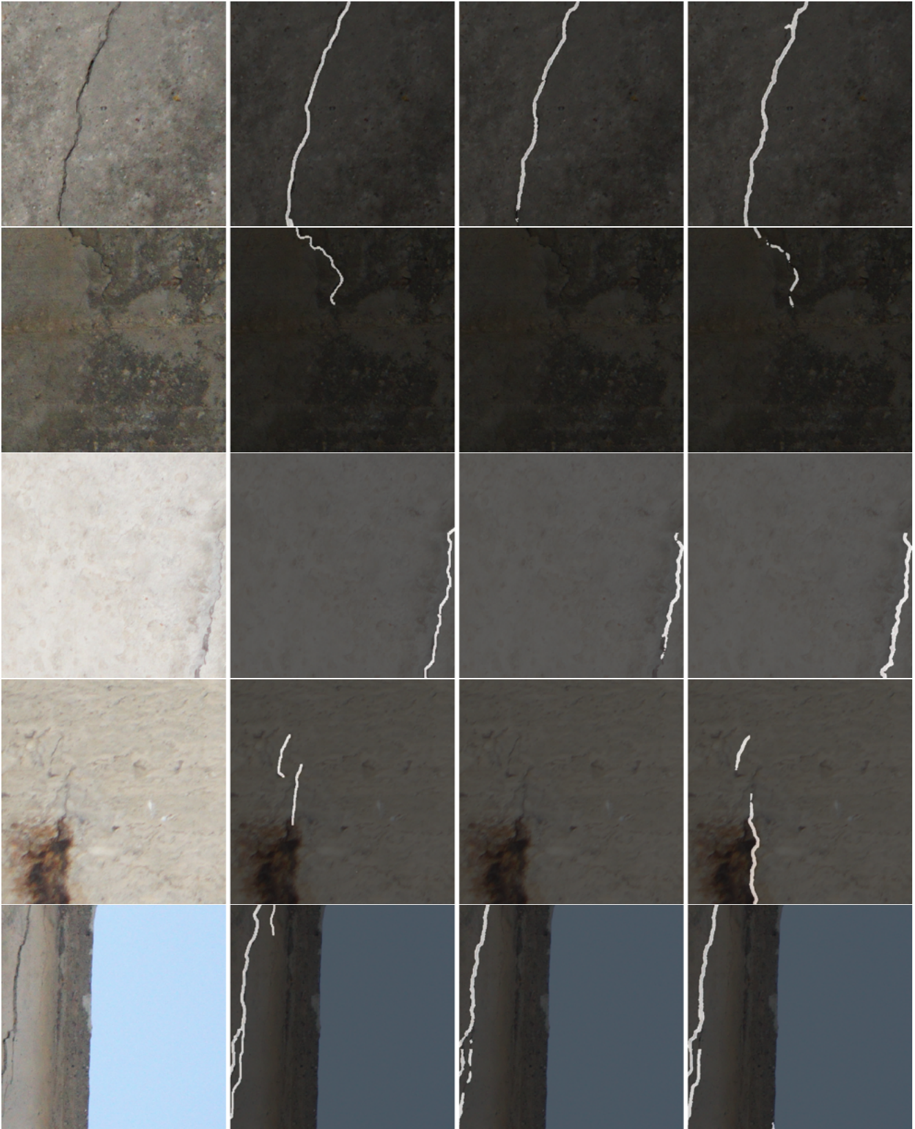
Figure 6. Qualitative examples on SegCODEBRIM from left to right: input image, ground-truth, U-Net, CAP-Net (ours). In general, CAP-Net segments cracks that U-Net often misses entirely. Images are compressed for view in pdf.
