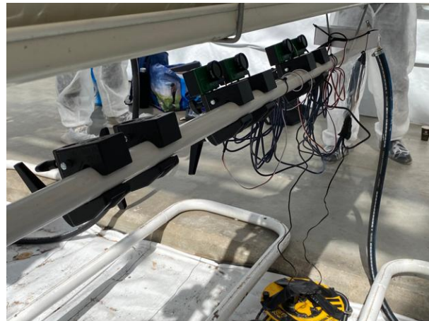
Figure 10. Camera installation for data collection. The cameras were fixed to the heating pipe and connected to the electrical grid with the yellow USB hub.
